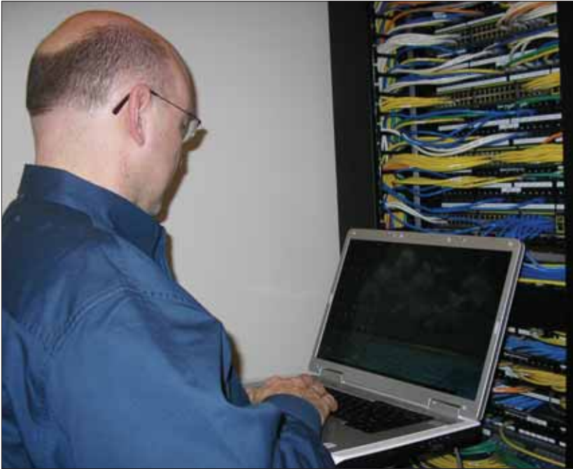
Greg Coon, service manager with ProTech Security of North Canton, Ohio, programs a fully IP-based security system that includes an S2 NetBox access control device using an ordinary LAN connection at Jackson High School.
